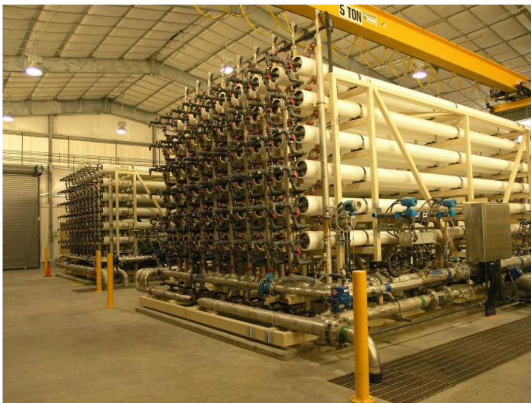
Figure 2-3. Two reverse osmosis treatment racks of the BCWTP. The white vessels in the racks contain the spiral-wound RO membranes. Each rack contains two stages: Stage 1 contains six columns of RO vessels, Stage 2 contains 3 columns of RO vessels.
