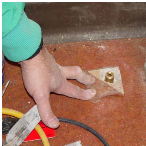
Figure D-4. Installation of subslab soil gas sample port. Courtesy Kansas Department of Health and Environment
