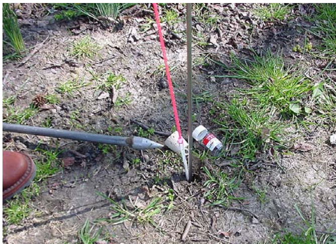
Figure D-3. Installing a passive soil gas module. Courtesy W.L. Gore & Associates, Inc.
